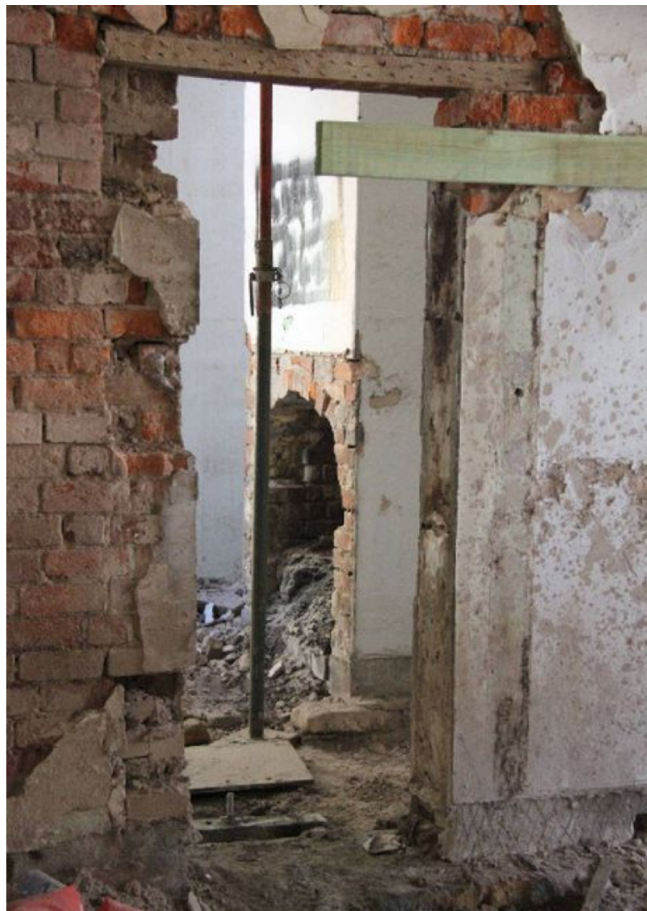
The internal rooms of the iconic building are severely dilapidated.
